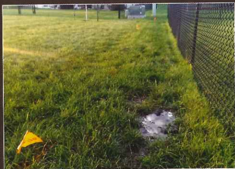
Lack of water infiltration
